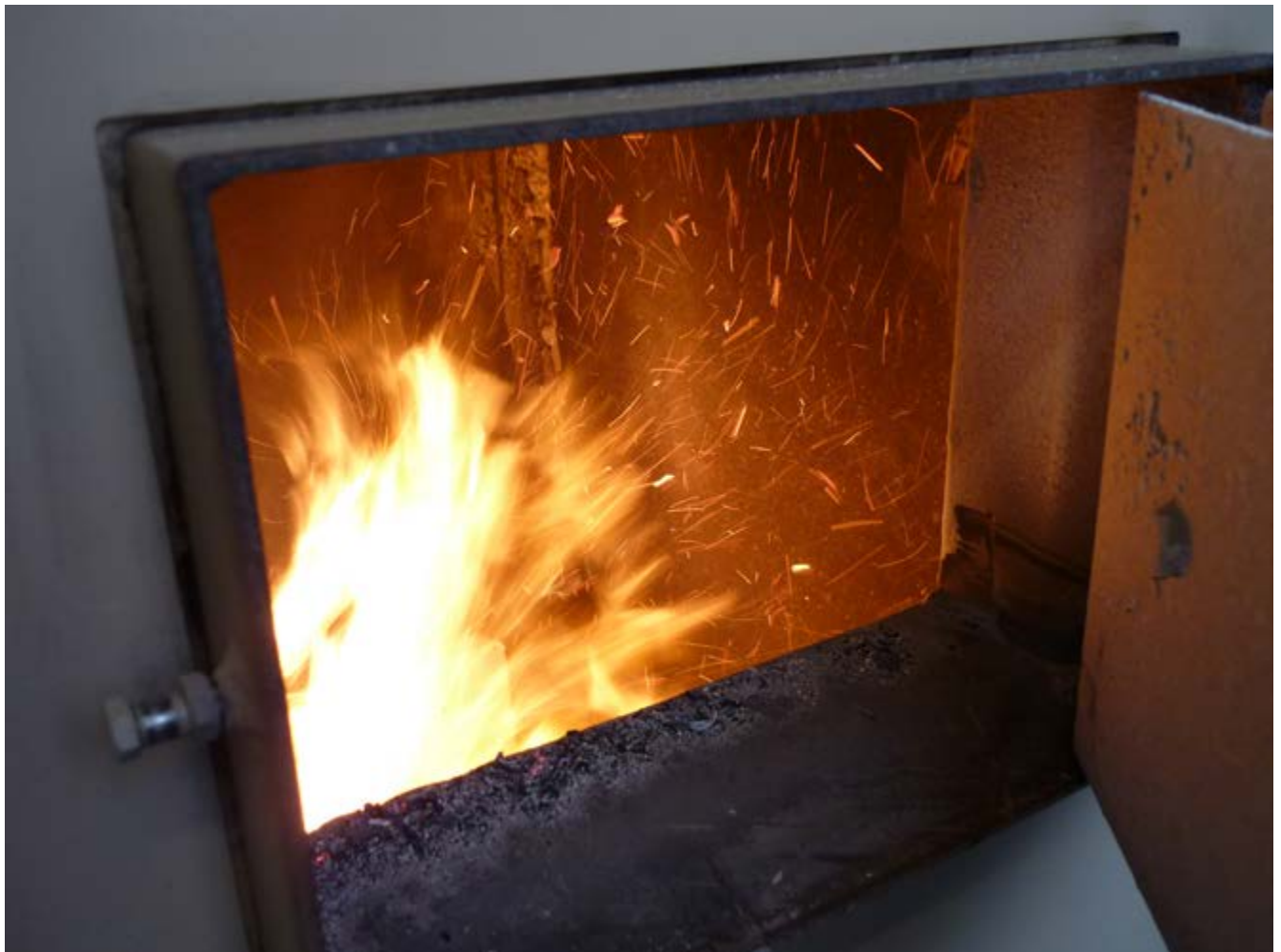
Combustion of willow, Veto boiler
